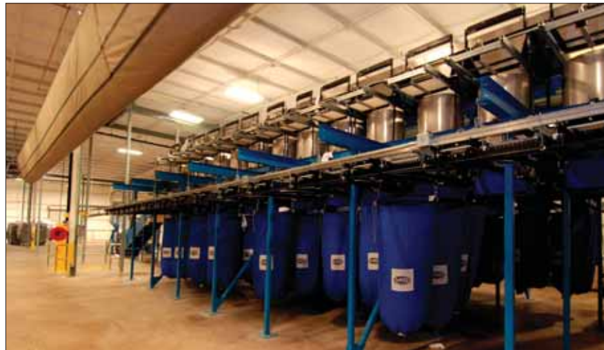
Boyd Gaming recently built a state-of-the-art green laundry facility in Henderson, Nev. that can handle 150,000 pounds of linen a day.
